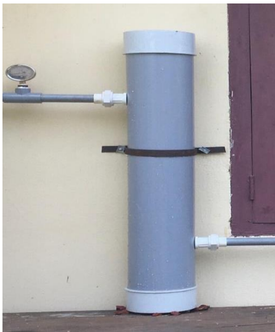
Fig. 1. Filter chamber fixed on the wall
